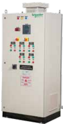
VarSet LV APFC panels without reactors
